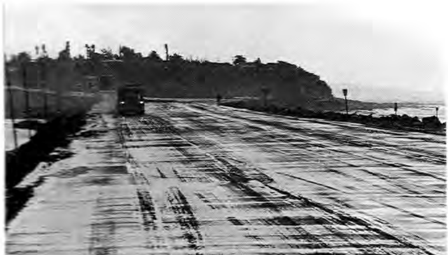
Aftermath of surf washing over Highway 101 in South Cardiff. Washouts along the highway are worsened by the loss of beach sand.
